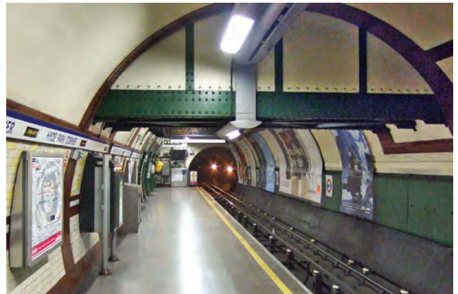
The subway bridge is seen crossing the westbound Piccadilly Line platform at Hyde Park Corner.
